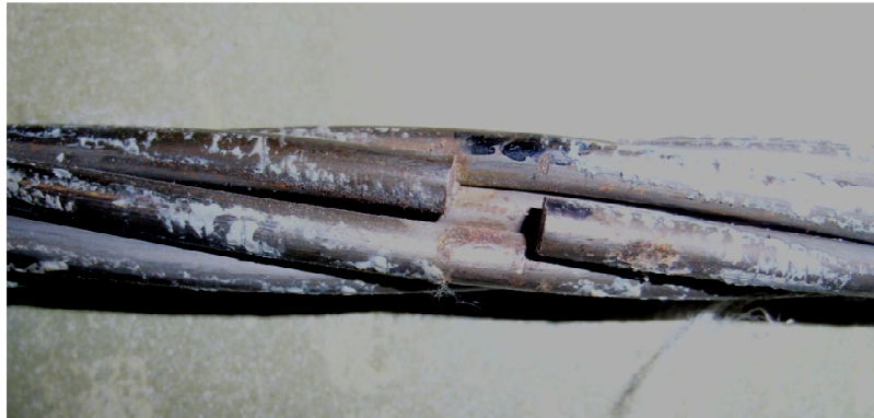
Figure 5.19 7-wire strand with one-broken-wire defect.
