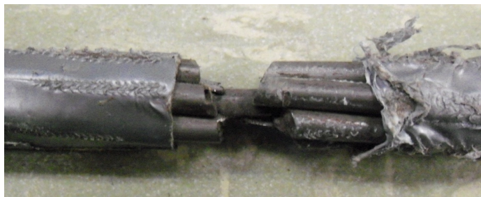
Figure 5.25 7-wire strand with six-broken-wire defect.
