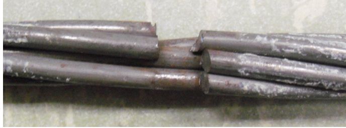
Figure 5.23 7-wire strand with three-broken-wire defect.
